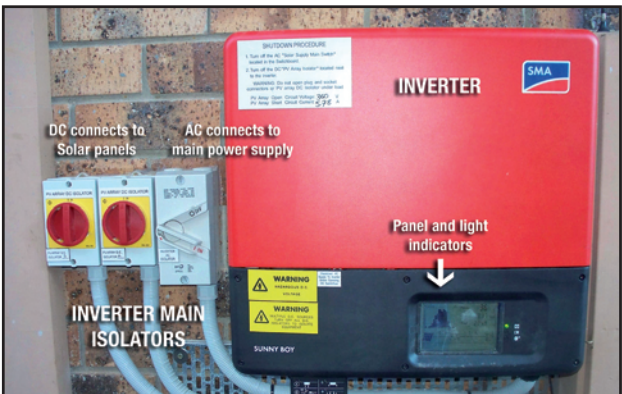
Figure 2 – Solar PV System
